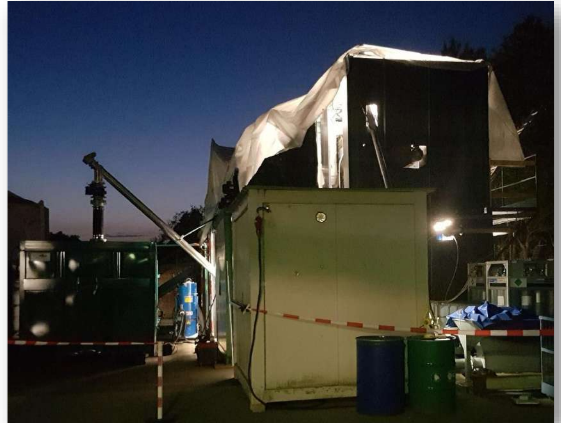
Commercial scale prototype for 7 t/day of sewage sludge in commissioning
